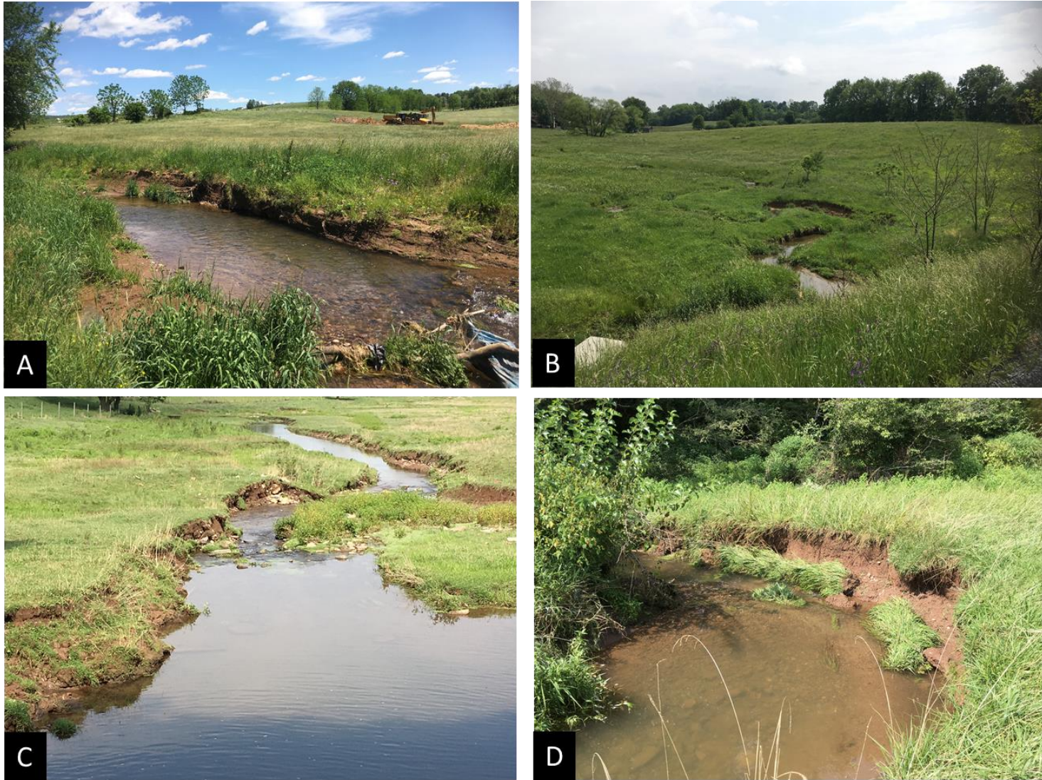
Figure 7. Example stream segments in the Hammer Creek Headwaters Subwatershed with obvious bank erosion and potential legacy sediment accumulations.
