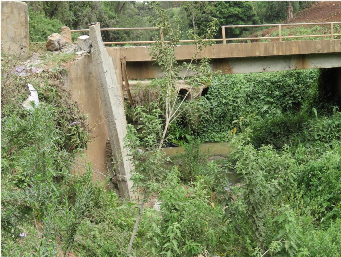
Figure B-1. Timau – CA01 streamgage from downstream looking upstream. This is after a car accident occurred so gauge housing is destroyed at the top. The flow at this section of the stream is typically low and heavily altered due to the culvert and bridge infrastructure present, and the riverbed is primarily bedrock in this section. Due to this, the streamgage was only able to monitor flows effectively during large rainfall pulses. Photo courtesy of author.
