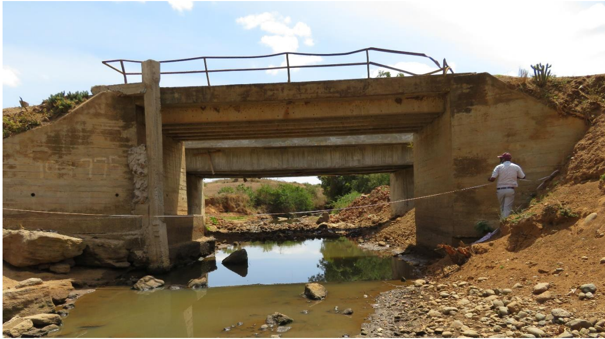
Figure B-6. Juakali – CA06 streamgage during low/no flow conditions. This gauge is located at a popular stream access point for the community, and therefore the banks and geometry at this location are heavily influenced by both the road infrastructure and the widened and less steep banks that have been carved out through access pathways. Once again, a pool is present under no-flow conditions. Photo courtesy of author.
