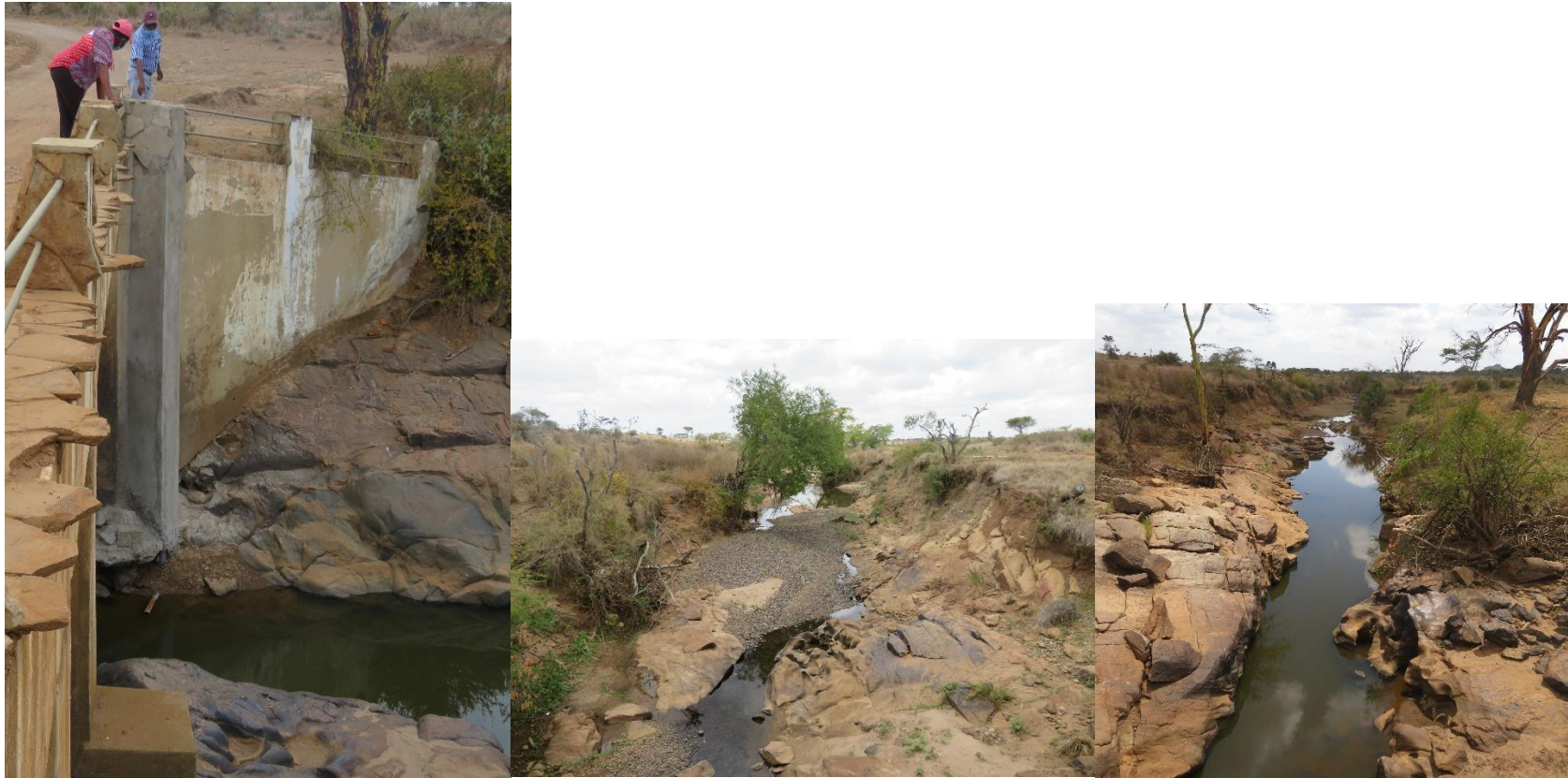
Figure B-8. Ol Jogi – CA08 streamgage during low/no-flow (left), looking upstream (center) and downstream (right). Looking closely the bottom of the gauge housing, the lateral pipe is visible above the water. Once again, the bedrock present at the site made installation difficult to capture very low flows, but at current levels the river barely has any flow. Photos courtesy of author.
